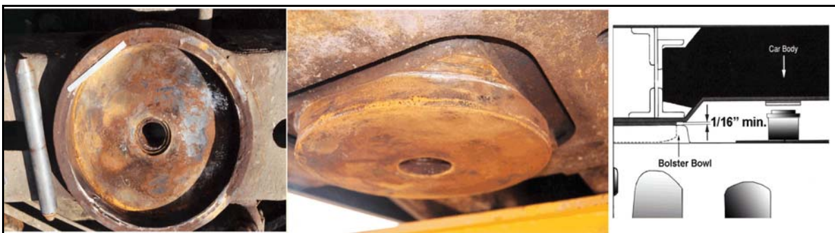
Photo 2. The truck bolster rim on car FURX 818699 was worn at four locations. The wear on the corners of the matching car body centre plate corresponded to the bolster rim wear. The sketch indicates the clearance between the two.
