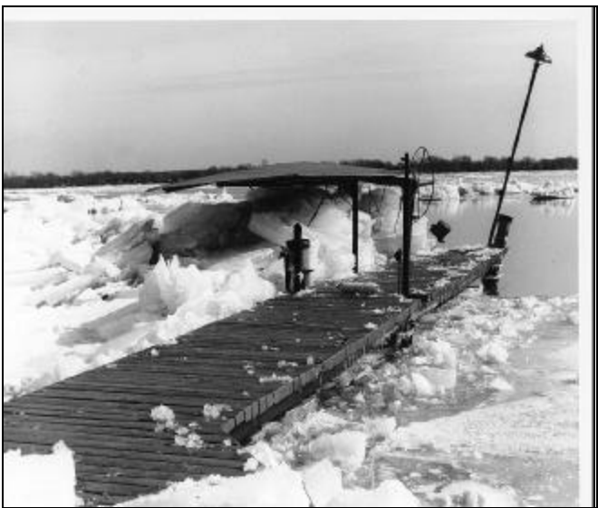
Ice damage to boat storage facility and dock in the upper Niagara River - 1955.
