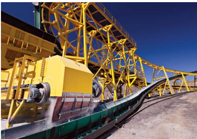
Vale’s New Demonstration Plant Featuring Canadian Innovative Hauling System Technology. Photo courtesy of Rail-Veyor Technologies Global Inc.
