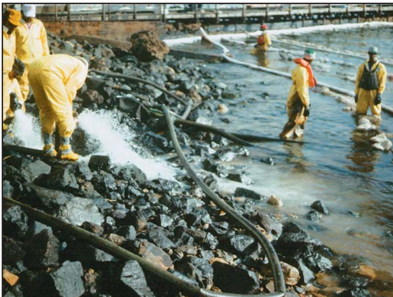
Figure 5.2 Flooding using hoses without nozzles.
