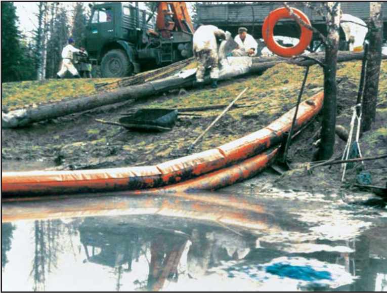
Figure 3.8 Shore-seal boom deployed across the waterline acts as a barrier to alongshore movement of oil.
