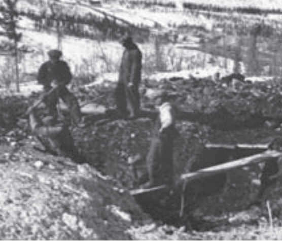
Digging through overburden (surface gravel) to test a buried vein, above the future Elsa townsite.
