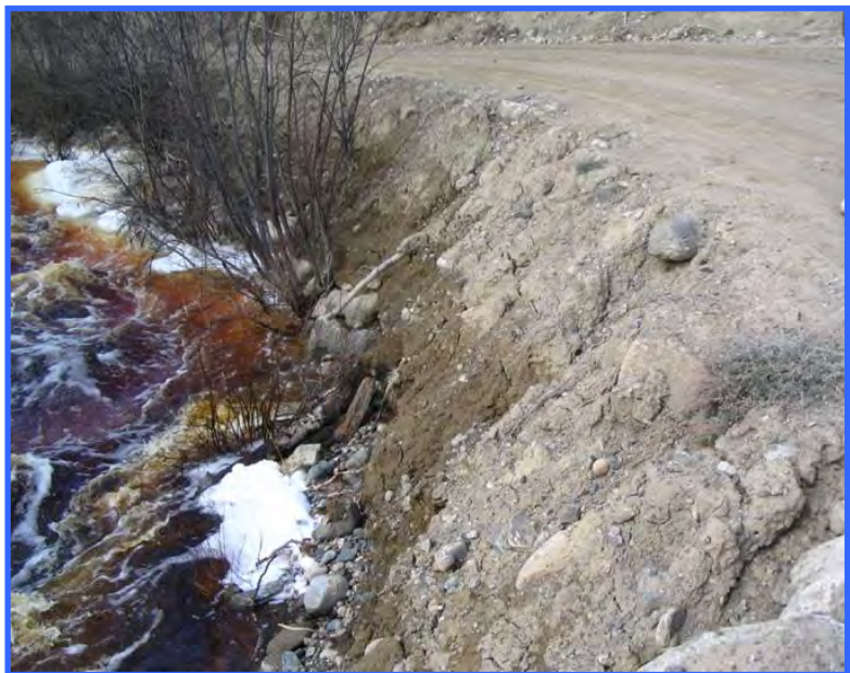
An unprotected stream bank that is being eroded by high water.
