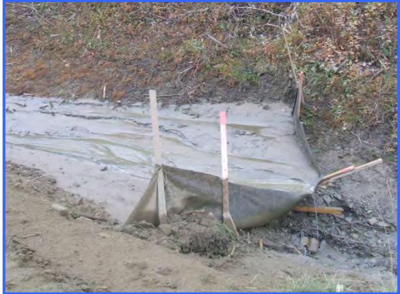
This silt fence illustrates that even an imperfectly implemented sediment control measure is better than nothing. The fence did its job, but could have been built better and it is beginning to fail. It is collapsing because of inadequate staking; metal rebar or larger wood stakes should have been used. Woven geotextile should have been used instead of unwoven, as it is stronger and will sag less. The fence will need to be cleaned out before being repaired or removed.
