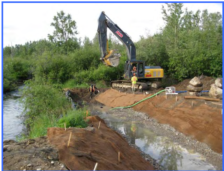
The project in this photo and the following photos involved lengthening two existing culverts at Watson Creek. To complete the work, the creek had to be diverted so the culvert extensions could be completed in the dry. This photograph shows the diversion channel on the right and Watson Creek on the left. The banks are lined with jute fabric to protect them from erosion. The new channel is being washed and the sediment-loaded water is being pumped out into the vegetation.
