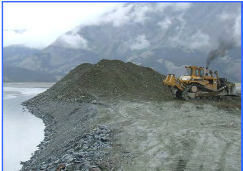
This stockpile of loose material should have been covered with plastic or geotextile to avoid sediment runoff into the river. Depending on how and when the material was to be used, it also should have been stockpiled away from the river.
