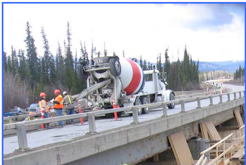
A sturdy work platform constructed below this bridge allowed easy access to the superstructure, but it also helped catch debris and keep uncured concrete from falling in the water.
