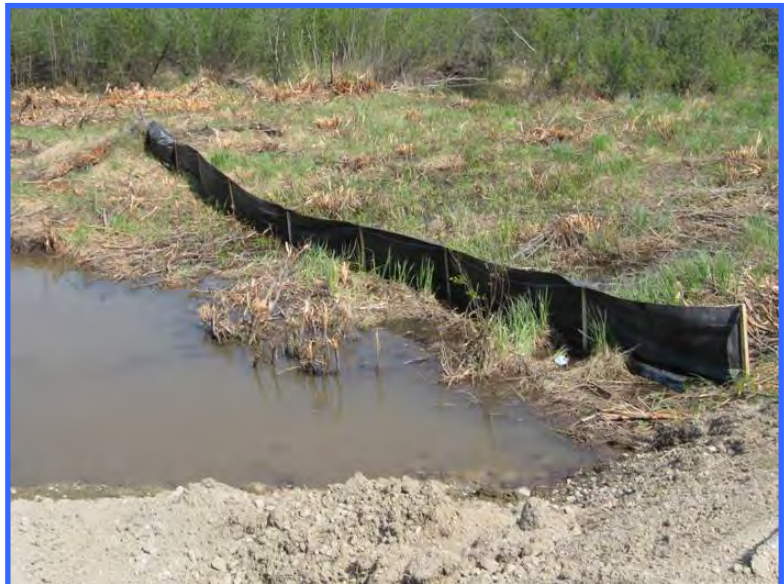
This silt fence should have been installed at the bottom of the disturbed slope rather than in the undisturbed vegetation. Currently it is non-functional.
