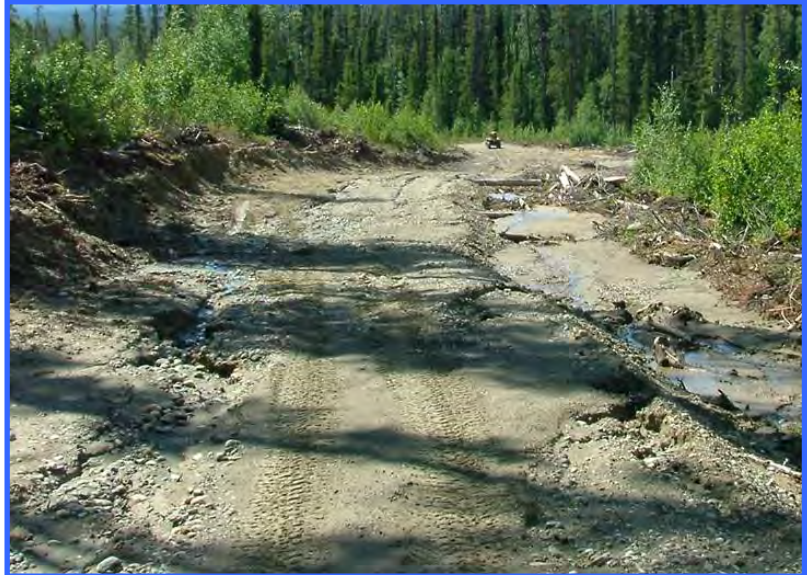
The lack of drainage control on this road has resulted in major washouts and has made the road barely useable.
