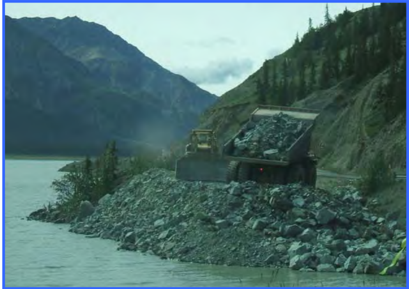
For this road-widening project, the lake edge had to be infilled. The procedure involved dumping rock on the ramp and then carefully push it into the lake with a dozer.
