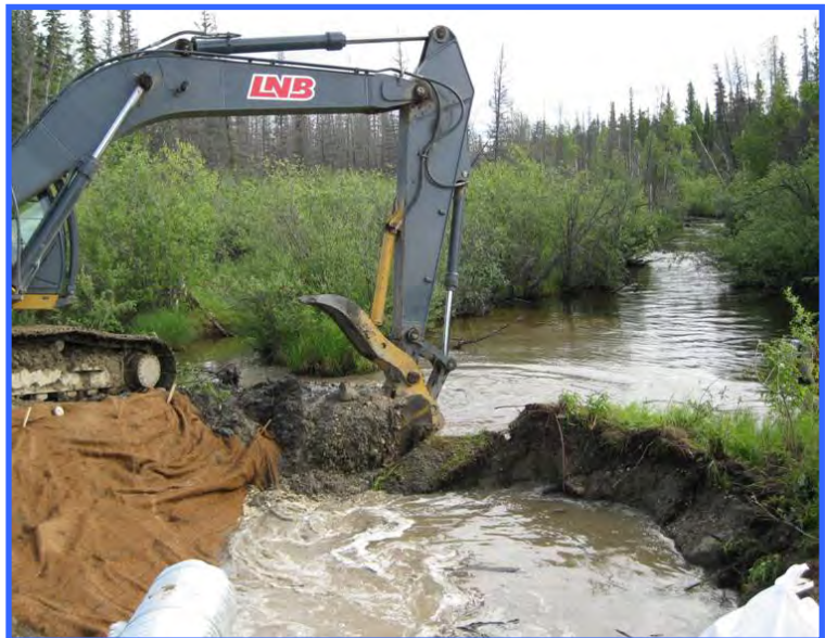
The same site as above. The upstream earth plug is being removed.
