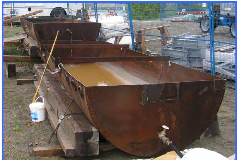
Creative use of an old tank as a sediment settling system. The upper container receives the sediment-laden water and has a passive overflow to the lower container, which has an outlet controlled by a valve.
