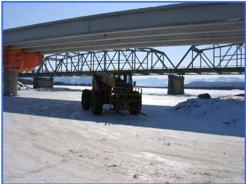
Working from the ice is often the best way to access the underside of bridges, and makes it much easier to protect water bodies. In this case, an ice bridge across the Donjek River was built to facilitate construction of a new bridge.
