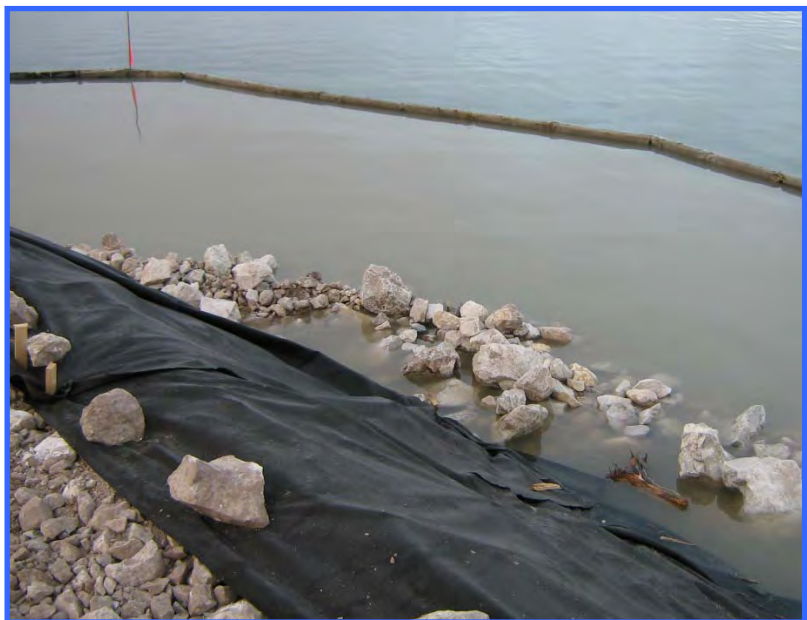
Little Atlin Lake boat ramp is being expanded. Infill area in the lake has been isolated with a silt curtain to contain sediment. Note the turbid water inside of the silt curtain compared to the clear water beyond.
