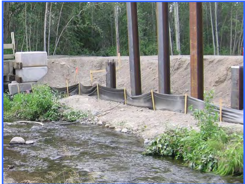
This silt fence was installed along a creek as a perimeter fence to keep loose material from rolling into the water.
