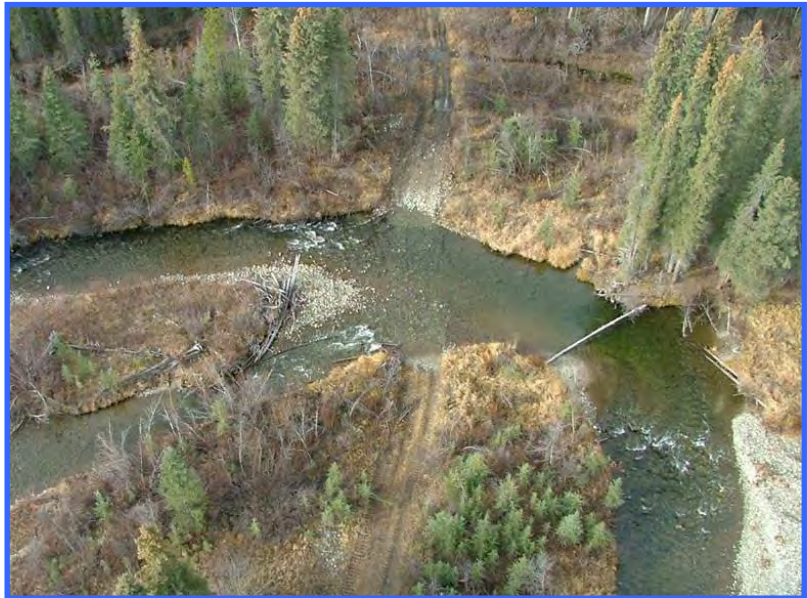
This type of stream fording is a thing of the past in Yukon, and never should have reached this state. There has obviously been many fordings over the years, leaving permanent marks in a fish-bearing stream. A temporary bridge should have been installed.
