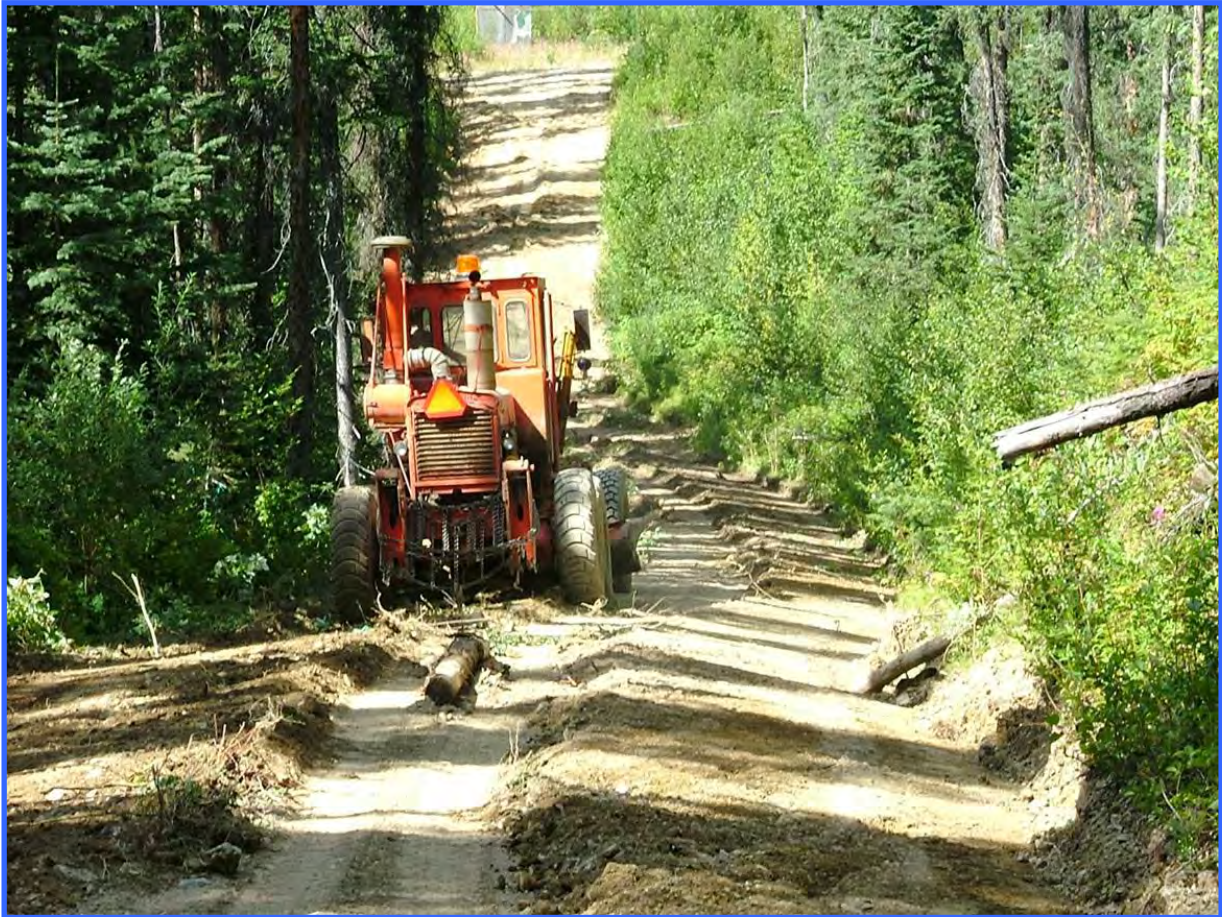
Proper sloping, crowning, and ditch placement on this road is creating good drainage and a stable roadbed.
