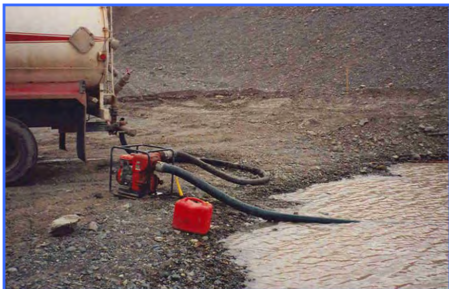
An unacceptable pump station. Water pumps need to be placed in spill trays and fuel must be stored >30 m away from any water body.
