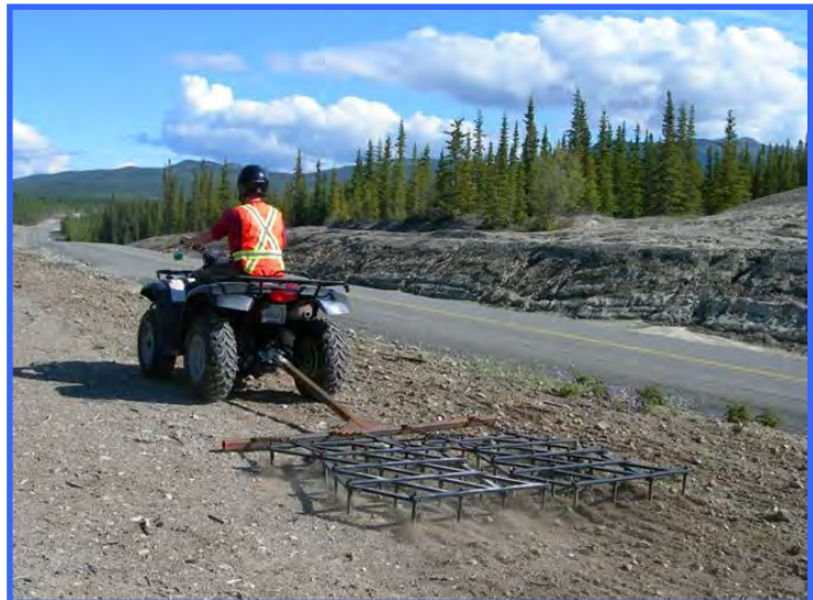
A harrow is used to loosen the surface soil prior to seeding. Seeding projects can often be completed by a two-person crew using an ATV equipped with a harrow and broadcast seeding, in conjunction with hand seeding.
