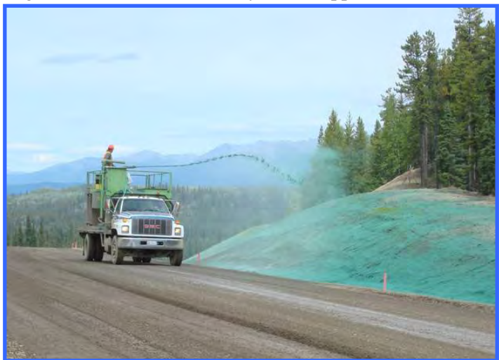
Hydroseeding in progress. A slurry containing fibrous mulch, seed and fertilizer is sprayed onto the slope to reduce erosion potential and promote quick revegetation. A tackifier is often included to hold the mixture together.
