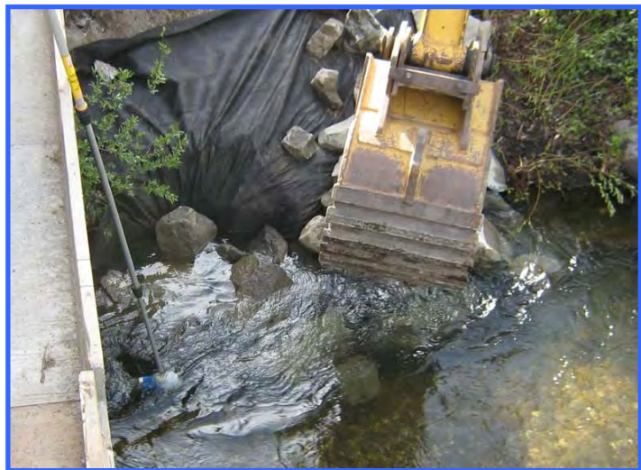
Careful placement of clean rock along a stream bank. A water sample is being collected to measure the turbidity caused by sediment release.
