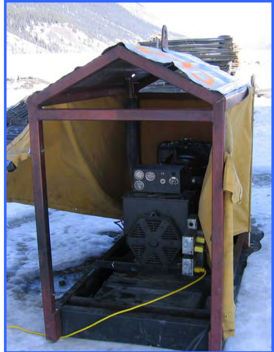
A generator properly set on a spill tray with roof and fabric to protect it from the weather.
