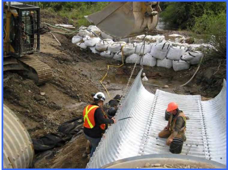
The same site as above. The work area is dry and the culvert extensions are being attached.
