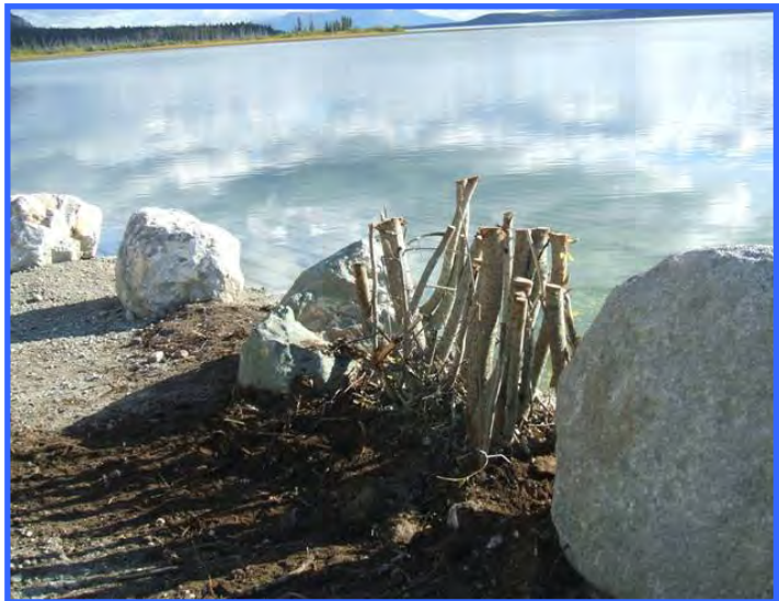
Willows are highly versatile shrubs that transplant easily if the roots are intact. This mature willow bush was cut off and then transplanted to a new location.
