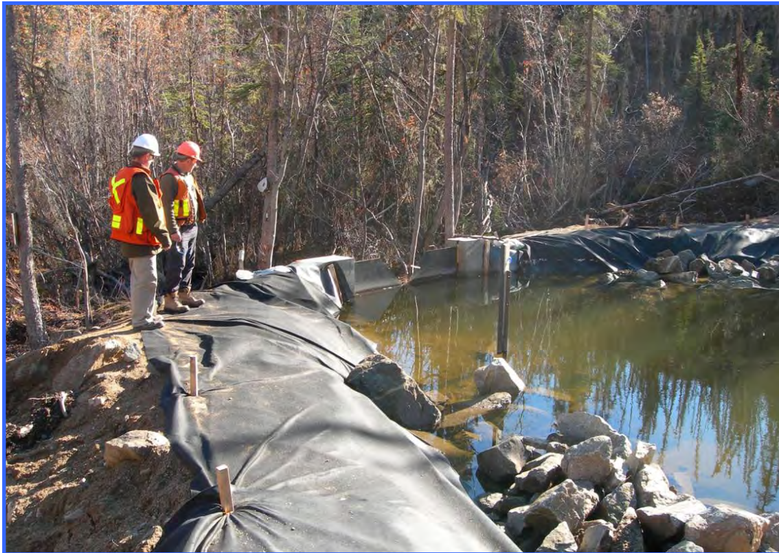
This is a well-designed and constructed sediment trap with a passive overflow.
