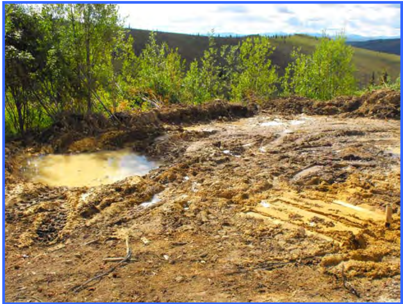
Decommission of this drilling pad is nearly complete. The sump is left and the site still needs to be reclaimed. Note the pile of organic material piled along the edge of the vegetation. This will be spread over the mineral soil and the site will be seeded.
