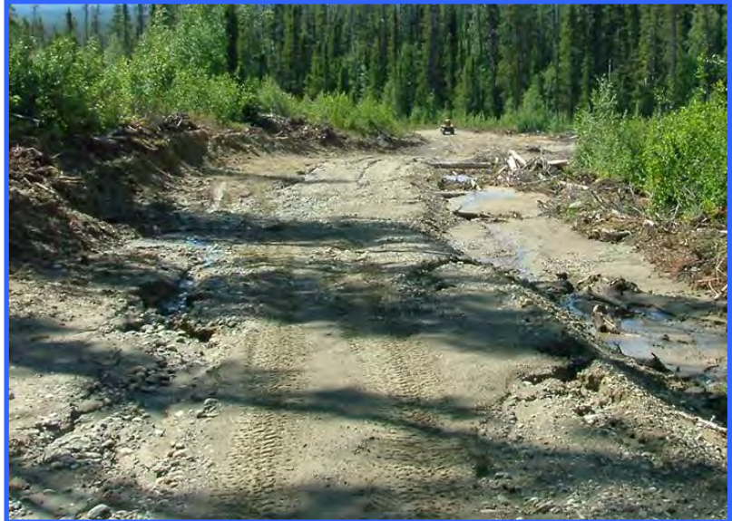
The lack of drainage control on this road has resulted in major washouts and has made the road barely useable.
