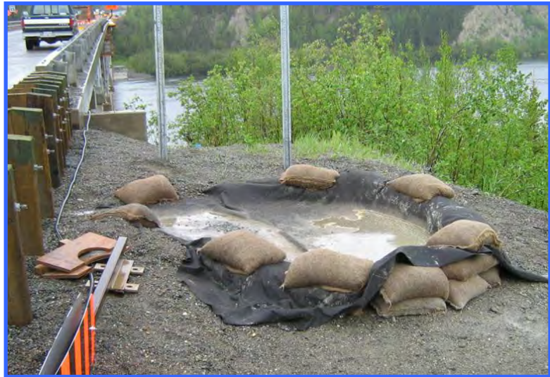
The size of a sediment trap depends on the volume of water that will be generated and sediment settling rate. This trap, while small, was built to contain a small volume of concrete curing water, and was adequate for the job.
