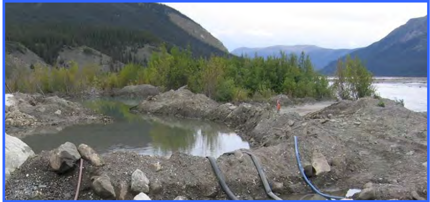
This sediment trap contains water pumped from isolated in-stream work areas created to construct a new bridge pier. This sediment trap has a passive overflow so clear water can exit the overflow and pass through vegetation before re-entering the adjacent stream.
