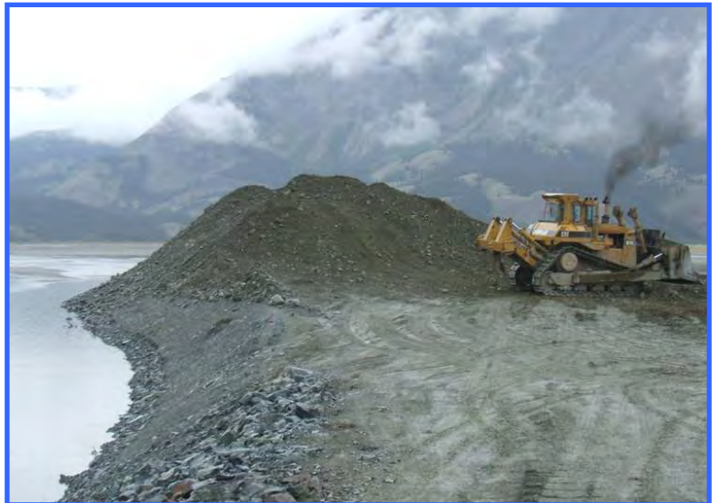
This stockpile of loose material should have been covered with plastic or geotextile to avoid sediment runoff into the river. Depending on how and when the material was to be used, it also should have been stockpiled away from the river.
