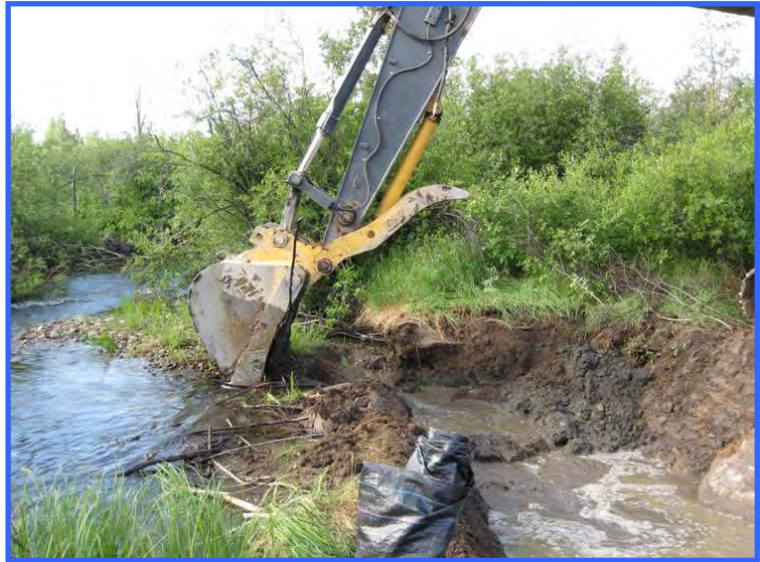
The same site as above. The downstream earth plug is being removed.
