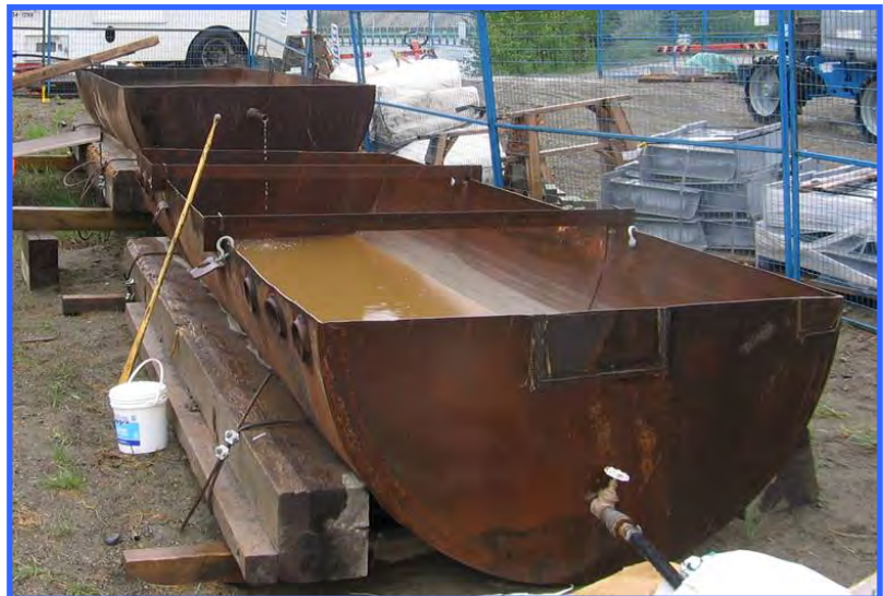
Creative use of an old tank as a sediment settling system. The upper container receives the sediment-laden water and has a passive overflow to the lower container, which has an outlet controlled by a valve.
