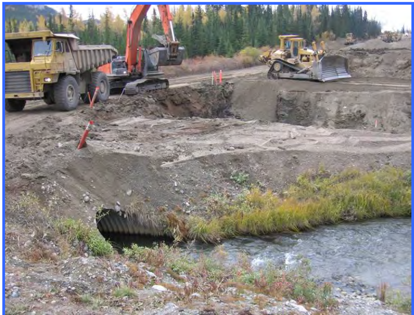
The site of a new culvert crossing is being prepared “in the dry”, while the stream is left undisturbed. The old culvert and channel will be reclaimed after the new one is activated.
