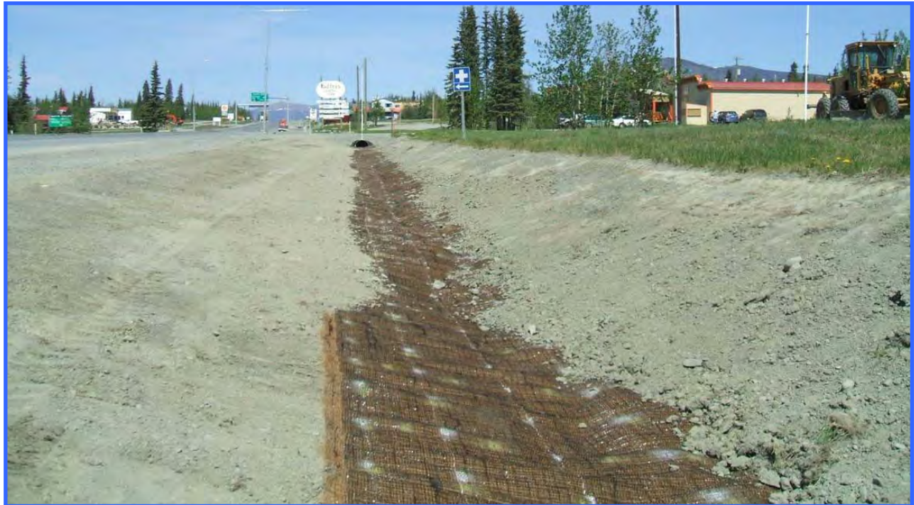
Coconut fibre matting reinforced with a UV resistant mesh was installed in this erosion-prone ditch that drained directly into an adjacent river. The site was seeded prior to installation of the matting. There are two installation errors to note: the edges of the matting should have been folded into the side slopes by means of an anchor trench, rather than lying flat on the ground. Also no dirt should have been put on top of the matting.
