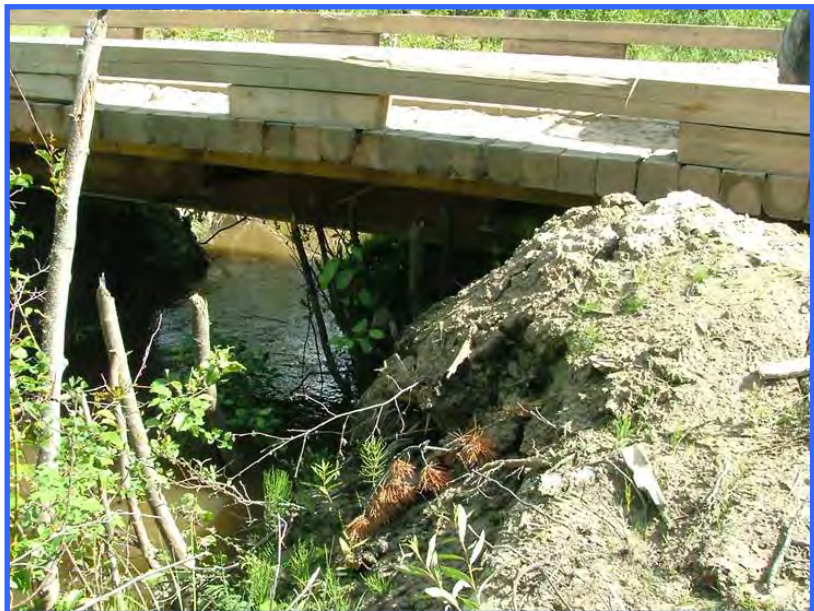
The abutment of this clear-span bridge should have been protected with riprap. Embankment collapse and sediment release are imminent.
