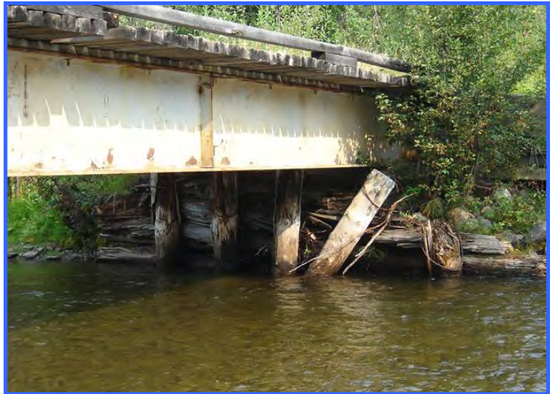
The abutment and approach (not shown) of this bridge failed because surface drainage water flowed to the bridge rather than being directed away from it. This could easily have been prevented with proper grading and bridge design.
