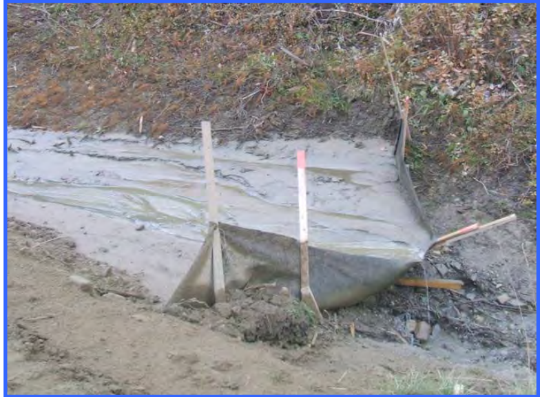
This silt fence illustrates that even an imperfectly implemented sediment control measure is better than nothing. The fence did its job, but could have been built better and it is beginning to fail. It is collapsing because of inadequate staking; metal rebar or larger wood stakes should have been used. Woven geotextile should have been used instead of unwoven, as it is stronger and will sag less. The fence will need to be cleaned out before being repaired or removed.
