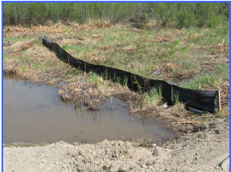
This silt fence should have been installed at the bottom of the disturbed slope rather than in the undisturbed vegetation. Currently it is non-functional.
