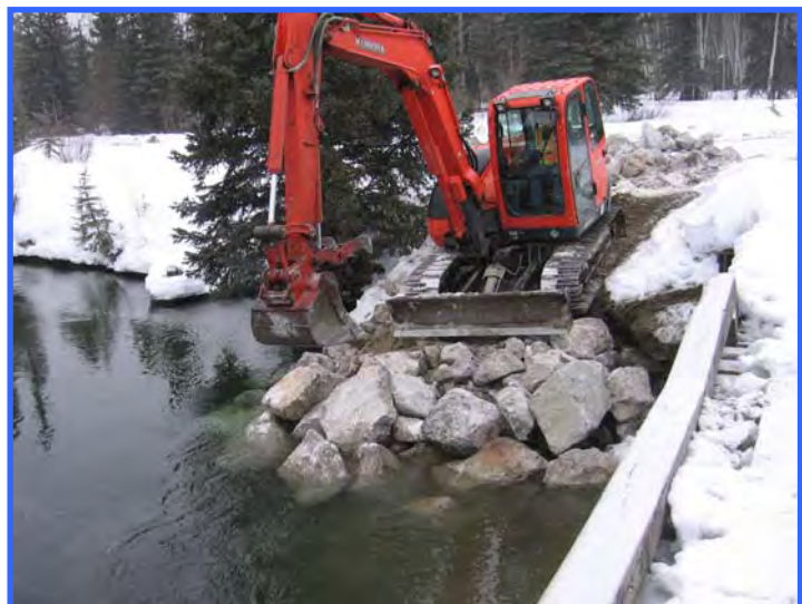
A temporary ramp consisting of large, clean rock infill was constructed so the excavator could access the stream and work underneath the bridge. After the work was completed, the rock was removed.
