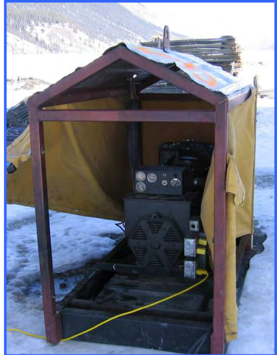
A generator properly set on a spill tray with roof and fabric to protect it from the weather.
