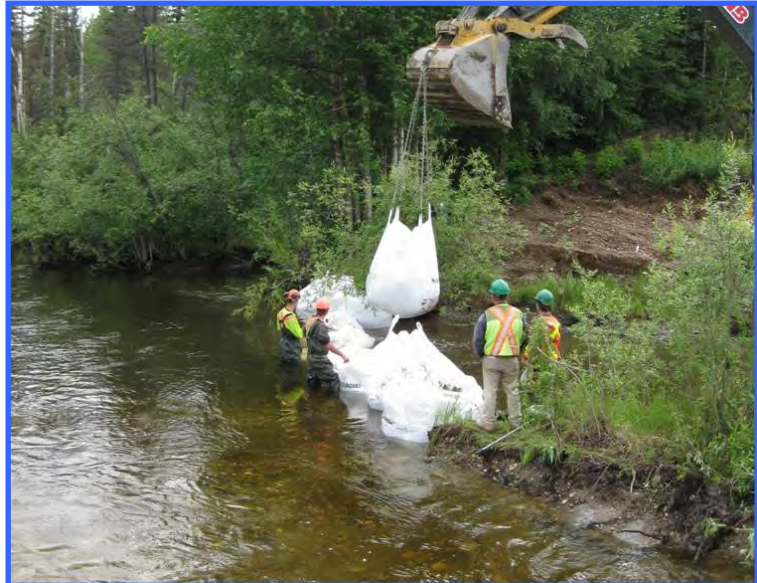
The same site as above. Watson Creek is being blocked off with large sand bags and the flow is captured by the diversion channel (foreground).
