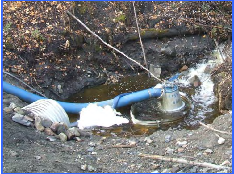
A pumped diversion showing the water intake. Even for this small stream, pumping its entire flow across the work site required large volume pumps.
