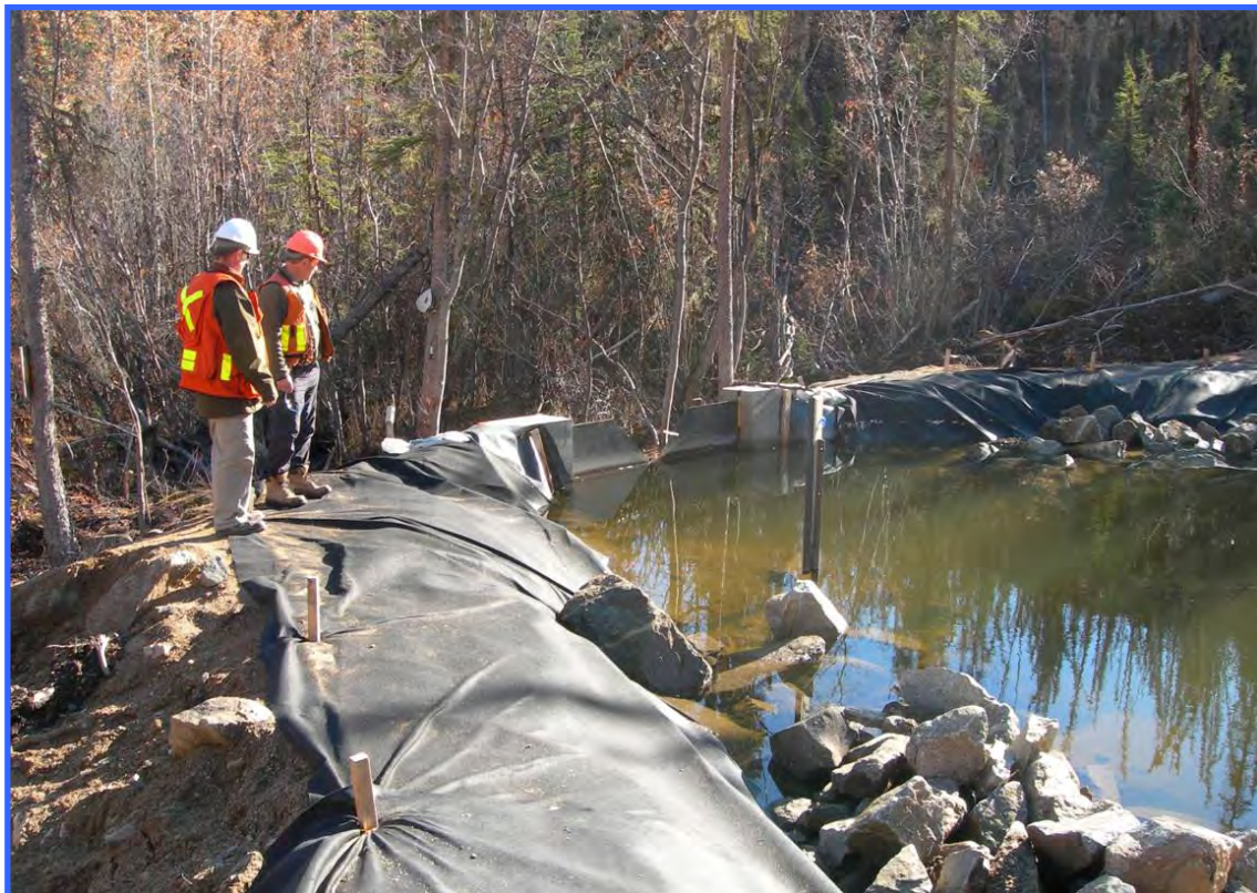
This is a well-designed and constructed sediment trap with a passive overflow.
