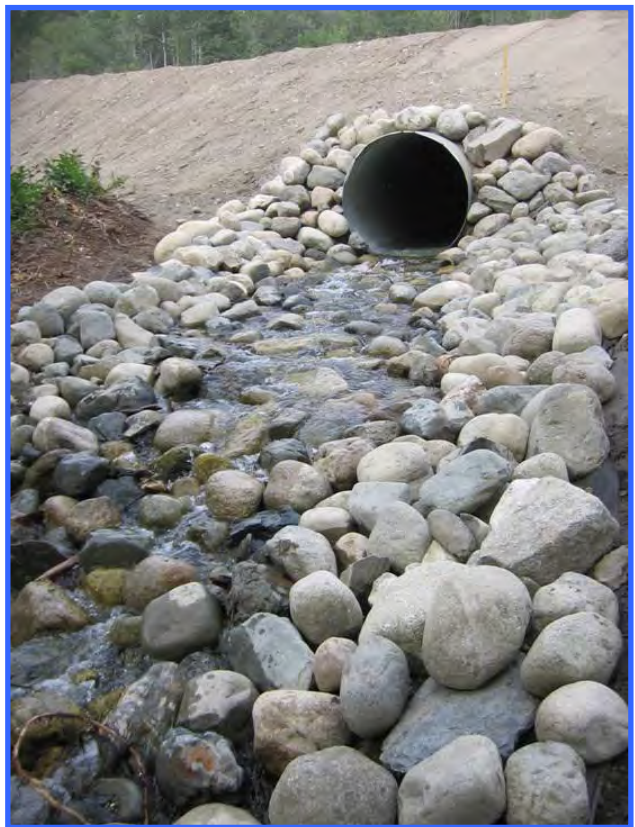
A rock flume is an erosion control measure commonly used for culvert outlets located on steep grades.
