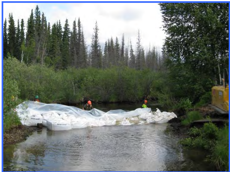
The same site as above. The sand bags are covered with plastic on the upstream side of the diversion. The plastic is anchored on the bottom with rocks to hold it in place and to seal the stream blockage.
