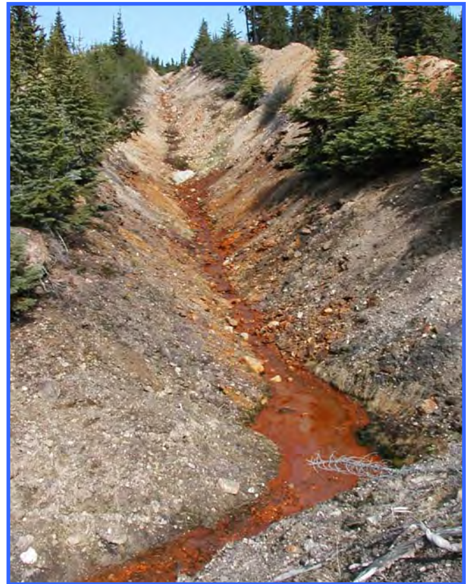
This exploration trench is cause for concern. The runoff is not being controlled and may be contaminated with heavy metals. The straight downhill run and slope grade mean that the trench should have been reclaimed, or at least stabilized (e.g., backfilled and vegetated).
