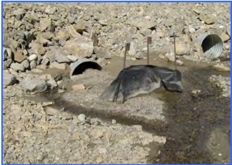
The attempt to keep this culvert (on left) from filling with sediment was too little and too late (the culvert on the right is only intended to be a high water overflow pipe). The silt fence is inadequate for the size and amount of sediment, and for high water flow velocities. The problem with two pipe systems is that the lower one fills with sediment during high water events if there is a lot of sediment flowing through the creek, such as this one. A much larger culvert should have been installed to avoid this situation.
