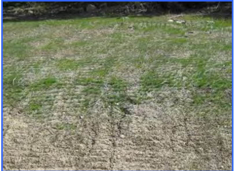
This slope was properly tracked with a dozer and seeded the year before this picture was taken.
