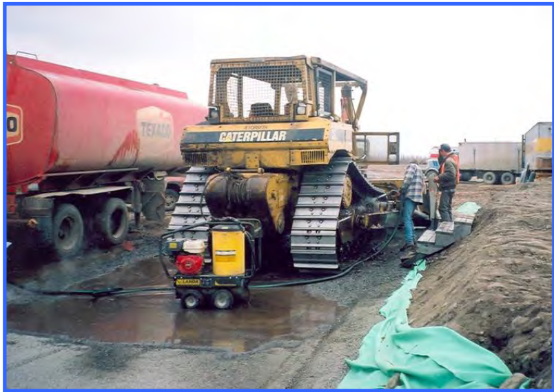
Pressure washing a dozer in a designated site that was lined and bermed.
