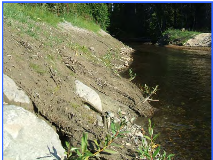
The same site as above one year later. Grass is emerging and the willow cuttings are growing along the water. The slope may look exposed and prone to erosion, but the buried matting is keeping the slope stable while vegetation becomes established.
