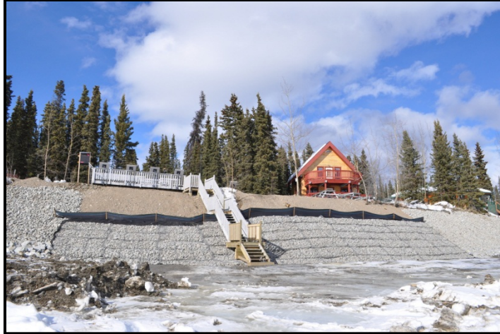
Figure 10. Erosion protection features at Swan Haven.
