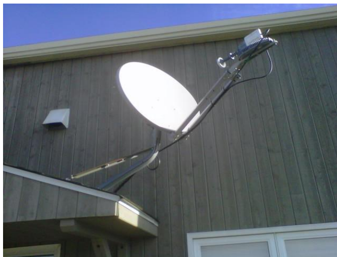
Figure 11.4: Direct-to-home Ka-band satellite dish
