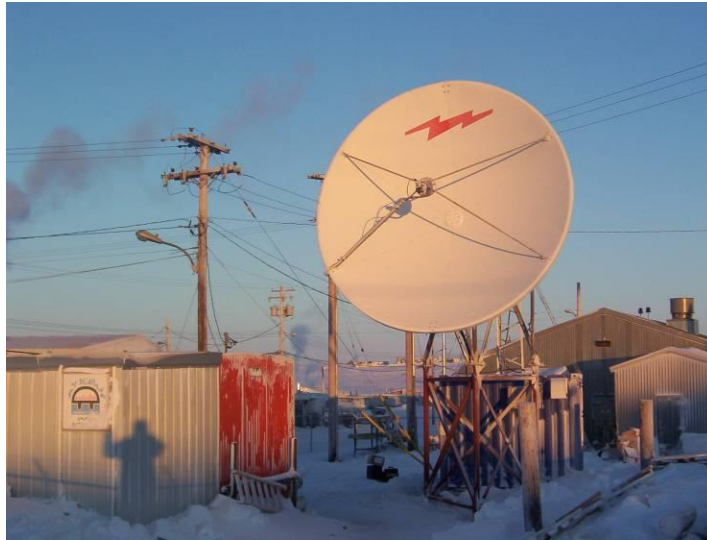
Figure 11.3: Community C-band antenna in Gjoa Haven
