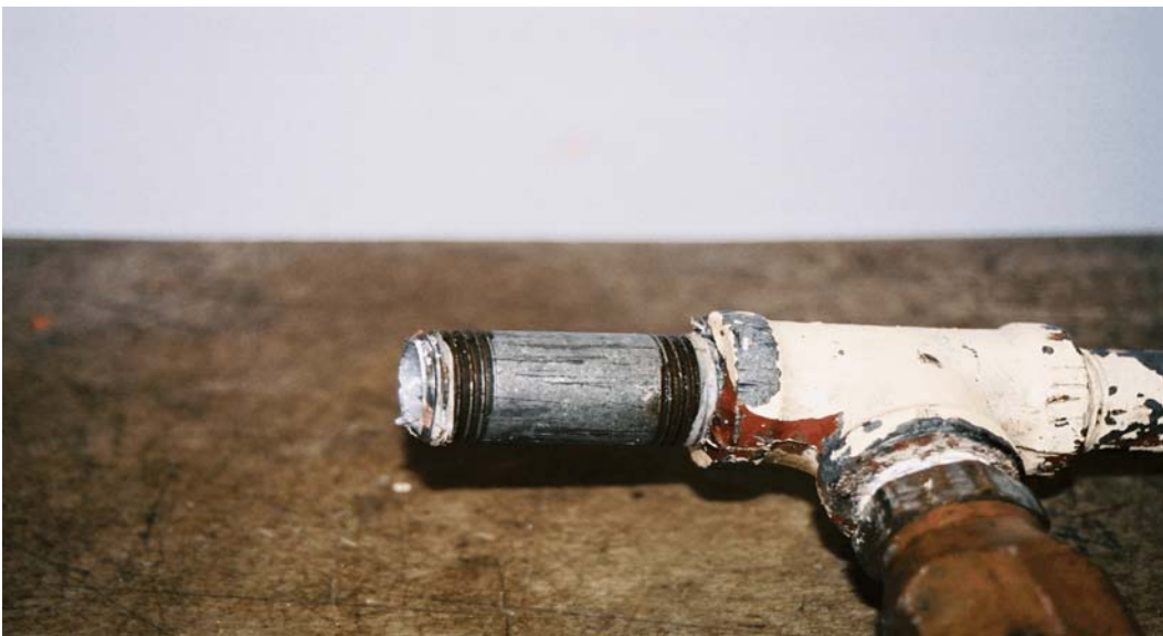
Photo 4. A fractured manifold pipe segment
