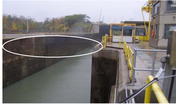
Photo 5. Daylight view of Lock 4's east chamber, with ship-arrester cable lowered in place (circled on the photo)
