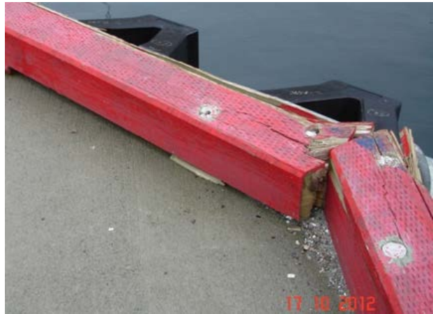
Photo 4. Damage to wooden cap rail
