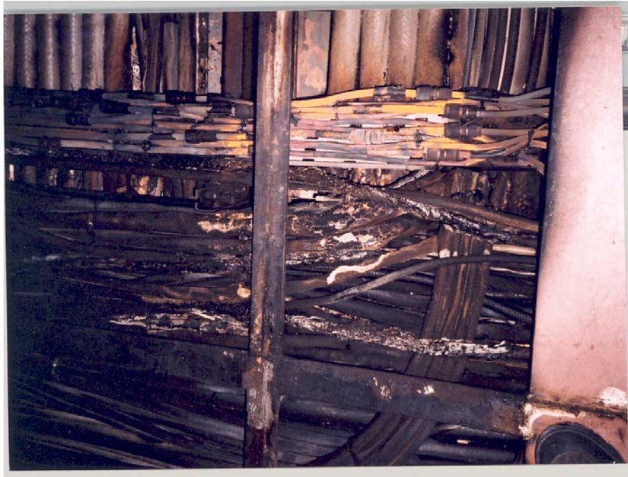
Photo 2. View of burned cabling above deck of engine control room (note effect of heat on copper tubing)
