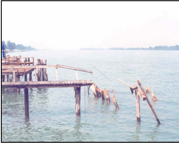
Photo 5. A damaged private dock
