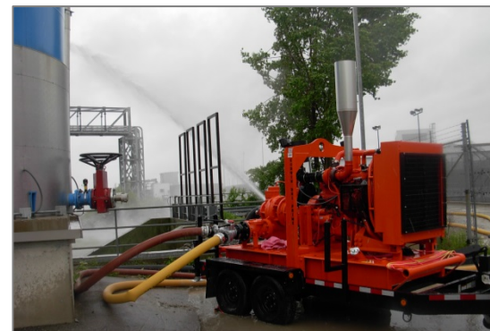
Darlington Emergency portable pumps further strengthen emergency preparedness.
