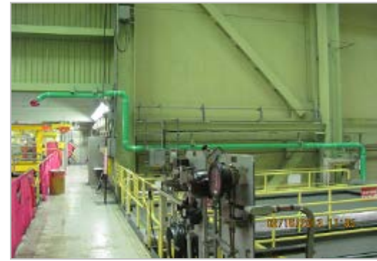
Permanent piping to spent fuel pool
