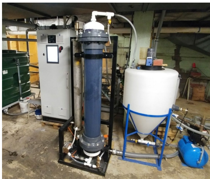
Figure 3: Greywater treatment system set-up used during the evaluation in Montréal.
