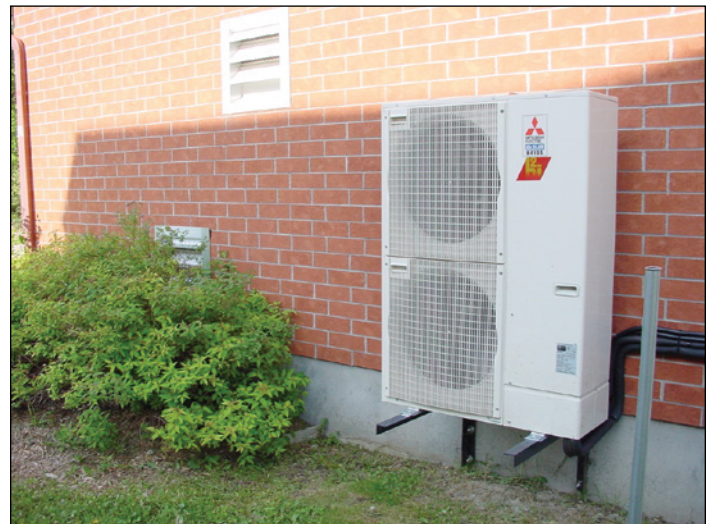
Figure 1 Outdoor section of the air source heat pump installed at the CCHT test house
